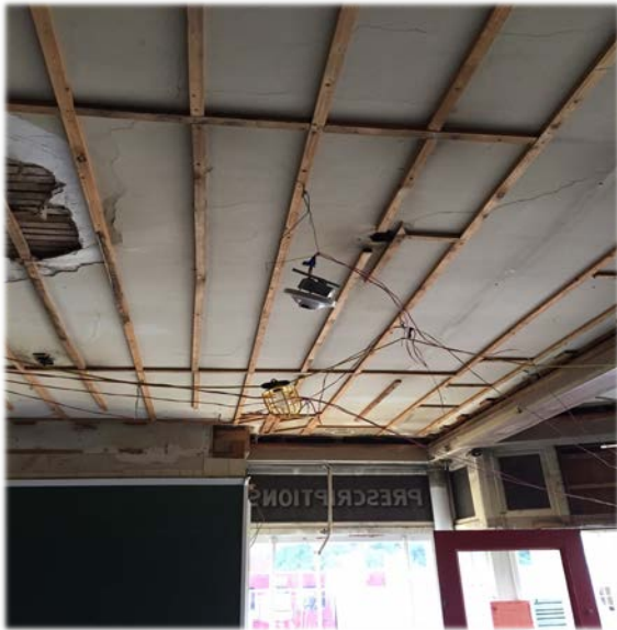
This smoke detector, hanging by its wires, is in the former Main Street Toy Shop. This space is being demolished for a new tenant. Much of the rest of the building was occupied at this time.
