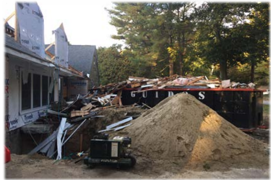
Residential construction site on Lexington Road. Violations of required construction site safety standards and Massachusetts Fire Code.
