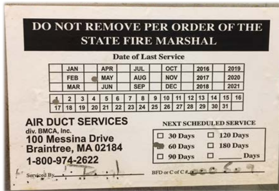
Discovered during an October 2016 annual liquor license inspection, this image is the cleaning and maintenance tag required by the Massachusetts Fire Code for a commercial kitchen hood. This was on a hood in a Concord Center business. It was three cleanings behind schedule and the grease buildup was a tremendous fire hazard. This hood requires cleaning every 60 days. Evidence that one annual inspection is not enough. They were ordered to correct this within 24 hours and they very willingly complied.
