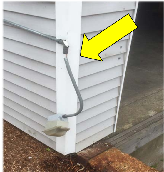
Front of 40 Beharrell Street. Exterior outlet pulled away from wall and hanging from conduit by its wires.
