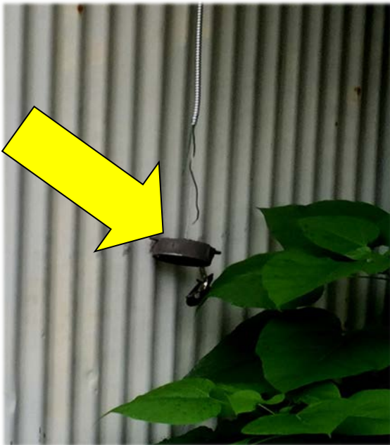
Rear of 40 Beharrell Street. Arrow is pointing to the hot and neutral electrical wires which are exposed. The electrical box is hanging from its ground wire. The wires were tested with a meter and they were live.
