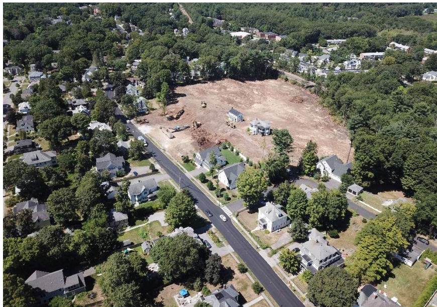
2025 aerial view of new subdivision construction on Main Street in West Concord, resulting in the demolition of two historic buildings and tree clearing (Doug Ellis)
