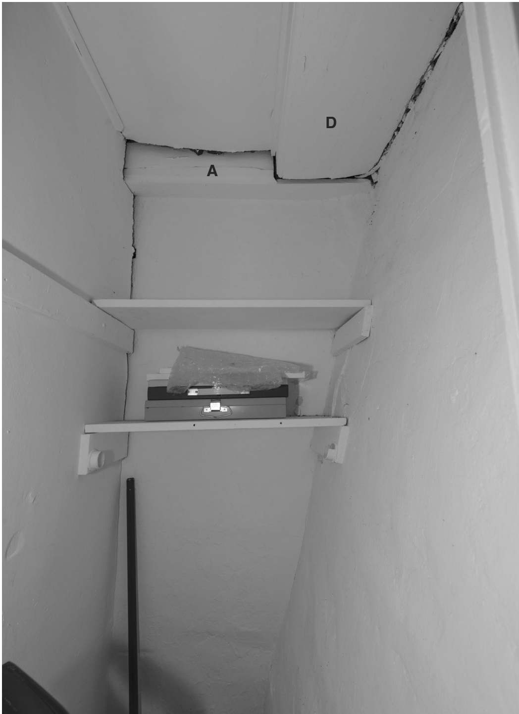
24.3: Room 203 - Fireplace Closet. Interior of the narrow closet next to the fireplace showing the joint of the original cased summer beam (D) to the original south wall girt (A). The wall appears to be separating from the summer beam. The plaster on the right is directly on the chimney masonry. All the plaster in the closet appears to be early.
