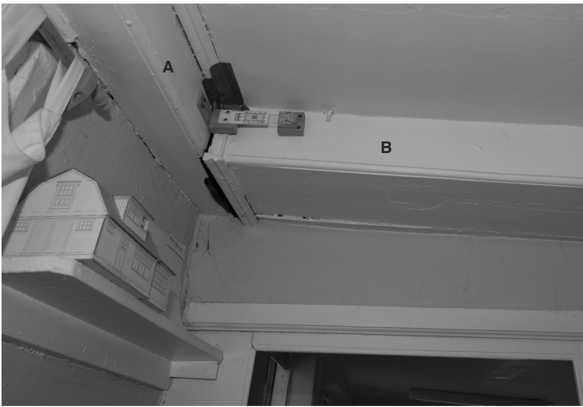
26.3: Room 207 - East Wall Detail. The north wall girt (A) appears to have pulled away from the casing of summerbeam "B".
