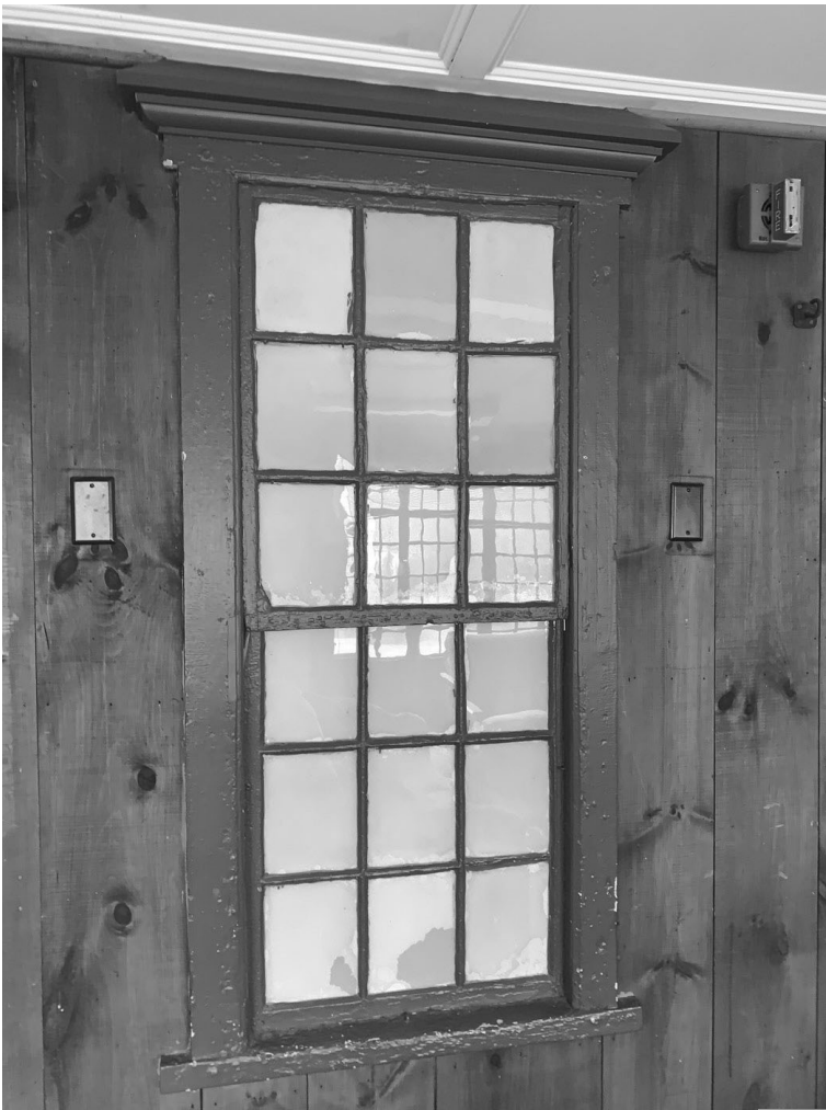
14.3: Room 105 - Bathroom. The exterior side of the early window in the south wall of bathroom 105 that was covered over by a recent renovation of the bathroom. This view is from within room 108.
