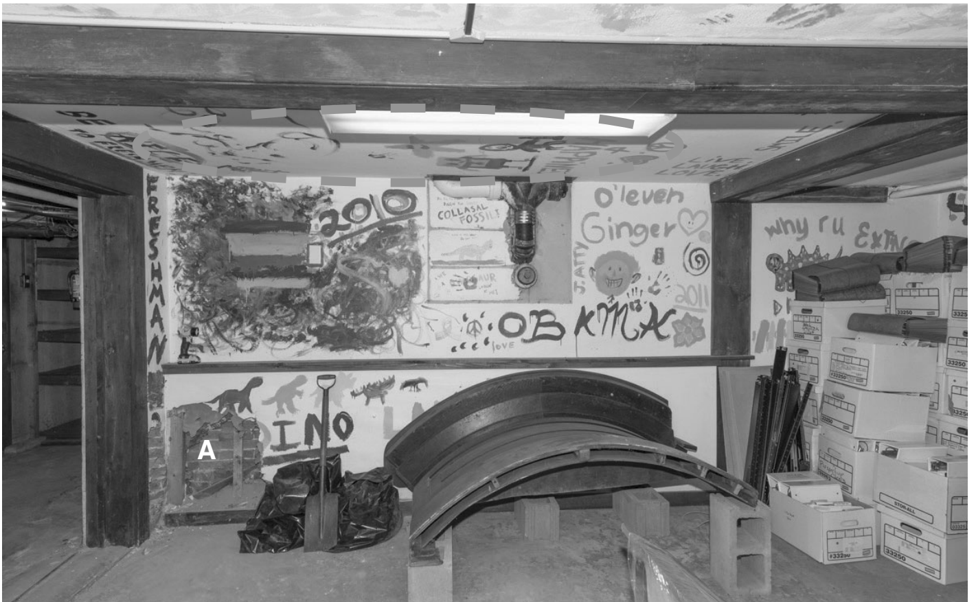
39.3: Room B03 - East Wall. This wall is the kitchen side of the ca. 1815 brick wall marked "A" in photo 37.3. The plaster covering the brick is modern, as is the woodwork forming the doorway and all the wood casings. As visible at "A", chronic rising damp has been causing the brick to spall. The area of the ceiling marked with the blue dashed circle is over framing that may have evidence for the location of the original chimney that was replaced ca. 1815 with the current south wall chimneys. This area is directly below room 100c in photo 5.1.
