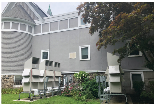
The condensers can extract hundreds of tons of heat every hour, even from frigid winter air.
