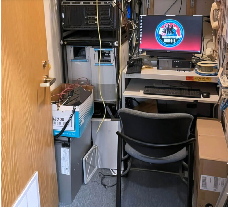
A police workstation crammed into a corner. Photo: Betsy Levinson/The Concord Bridge
