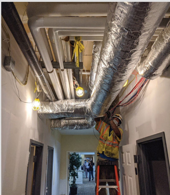
A worker installs insulated ducts at Concord Park. Insulation is key to a successful heat pump system.
