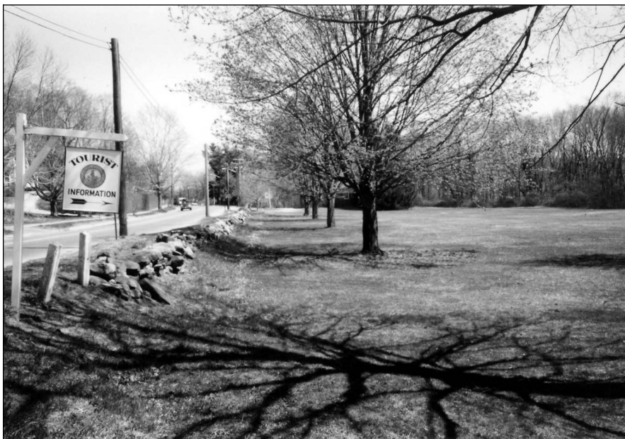
Figure 18. Circa 2002 view showing deteriorated condition of the stone wall along Lexington Road.
