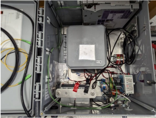
Figure 1: Advanced Metering Gateway
