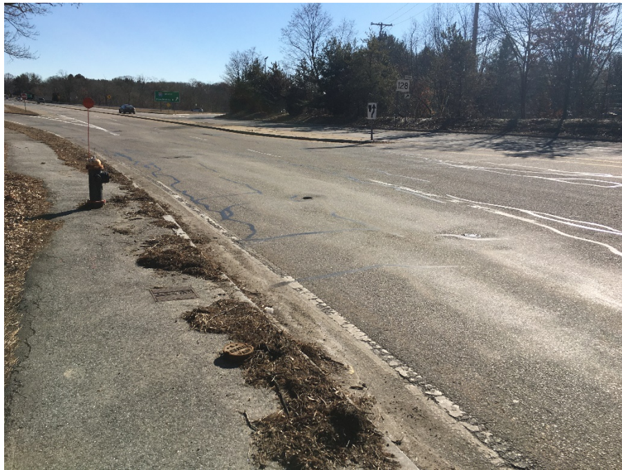
Overgrown sidewalk, deteriorating curb and pavement
