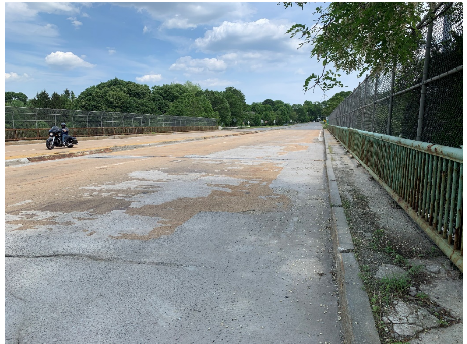
Deteriorating riding surface, rusting bridge rail, and settling sidewalk
