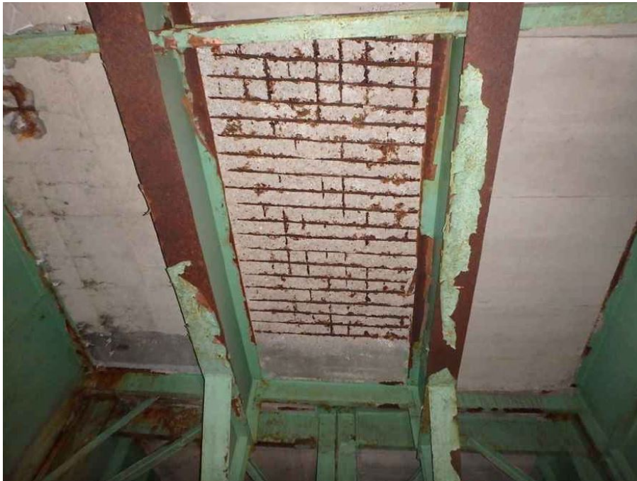
Deteriorated bridge deck & heavy rust on girders
