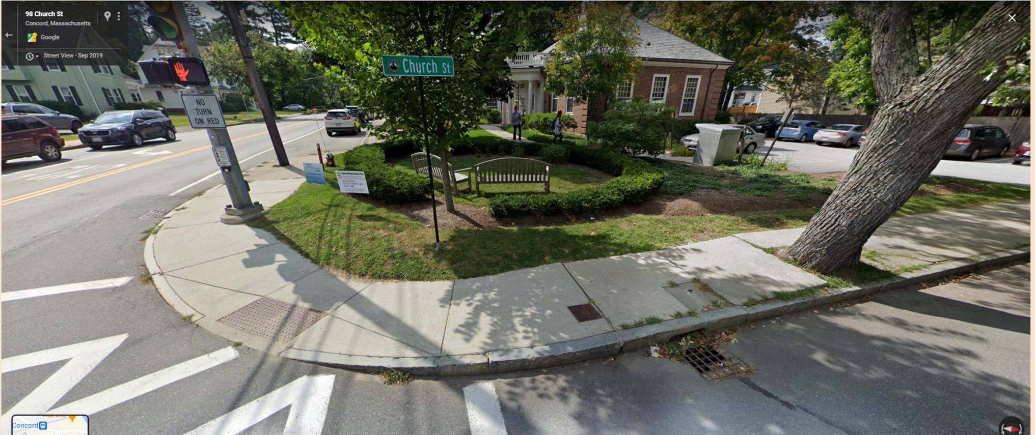
Another view of sidewalk issues in front of Fowler Library; it compromises peoples safe access to building; another area of concern w similar pole issues is Baker Ave; Concord Greens residents have long complained about that
