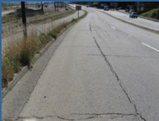
Longitudinal Cracks – High (>3/4")
