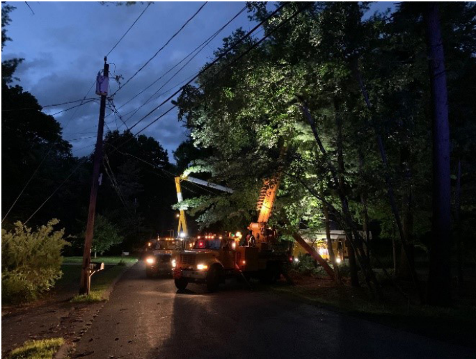
Emergency Response from August Storm
