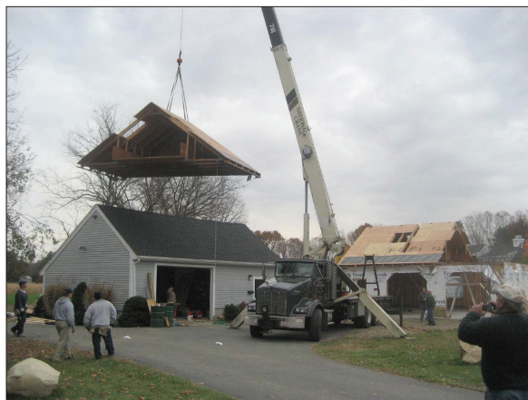
Nashoba Brooks School donated a garage which Jim Macone, with assistance of CPW team and prisoners from MCI, disassembled and reassembled at the Knoll for use of cemetery division activities.
