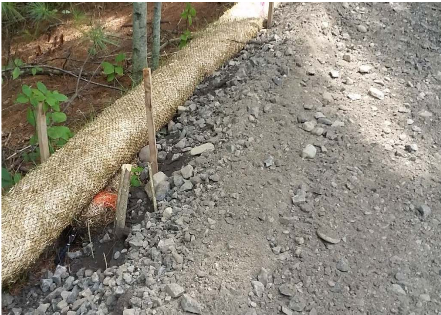
REPAIRED E/C AT EDGE OF SUBGRADE. SIMILAR REPAIRS ARE NECESSARY ALONG SUBGRADED AREAS.
