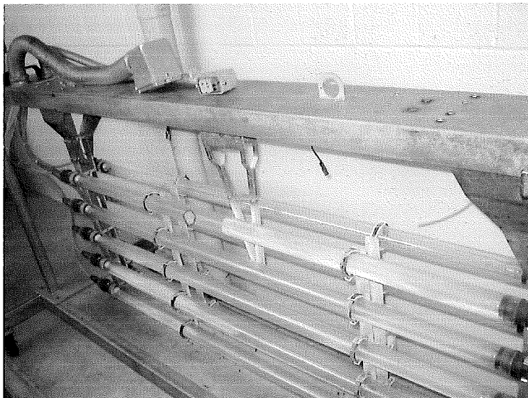
UV bank A module 1 in maintenance rack while plant staff repair the bulb wiper air cylinder
