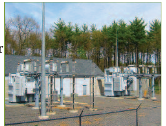
This West Concord substation will undergo improvements to increase its capacity.
