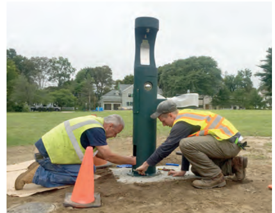
CPW Water Distribution Crew installing a water fountain with a bottle filler at the Alcott School.
