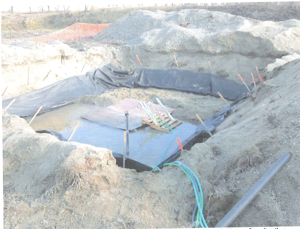
Hydrogeologic evaluation test pit in former intermittent sand filter #5 with 50 gpm flow distributor.
