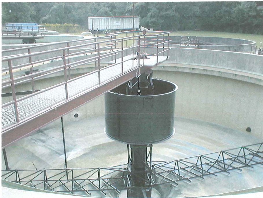
A view of the rehabbed #1 secondary clarifier prior returning to service on 8/27/11.
