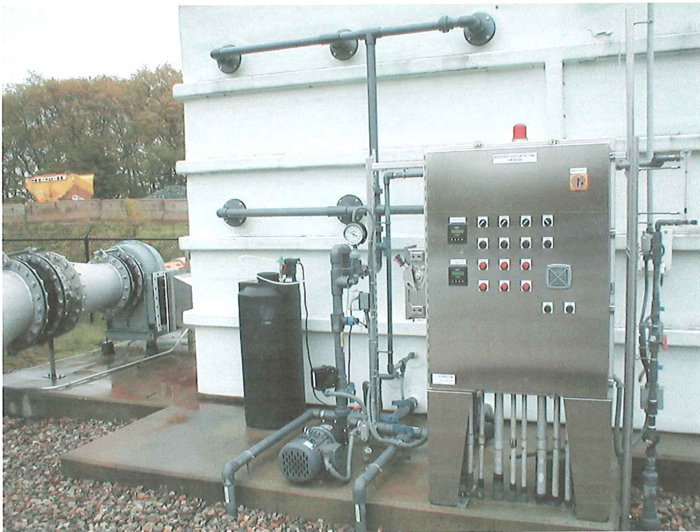
The odor scrubber resumed full "wet" operation in April with nutrient feed from drum on left and humidification water from plumbing on right.
