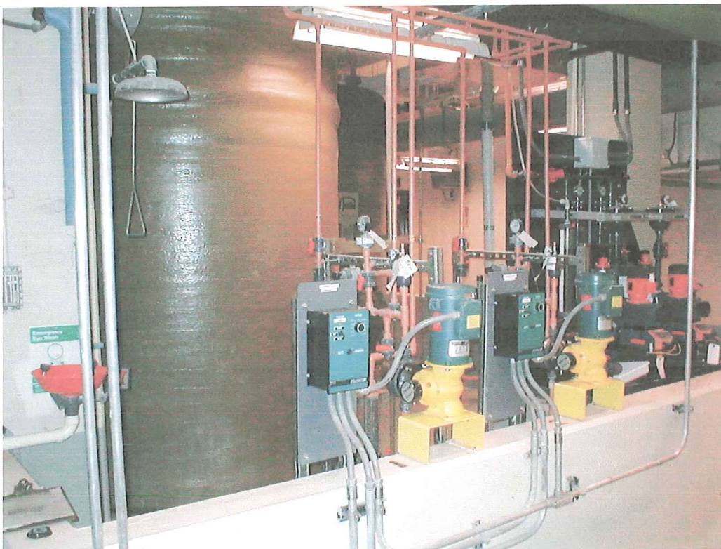
A view of the CWWTF aluminum sulfate (alum) bulk storage and pumping equipment.
