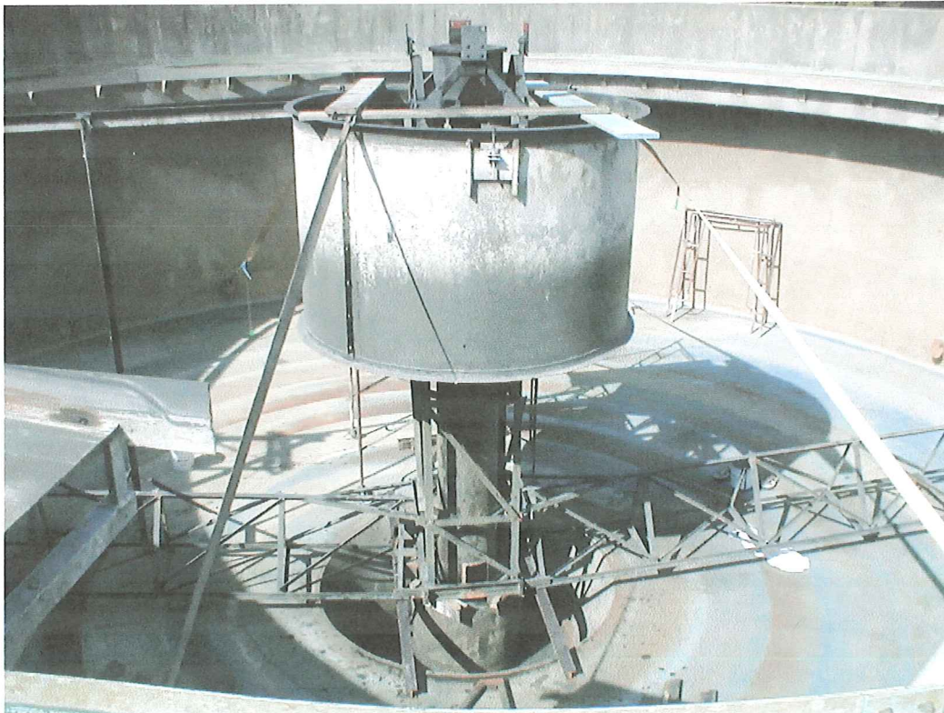
The #1 secondary clarifier with bridge and drive removed and ready to cover for sandblasting & painting.
