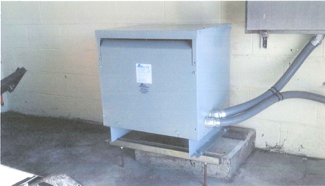
Newly Installed Transformer.
