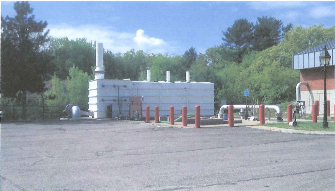
Concord WWTF odor control system.
