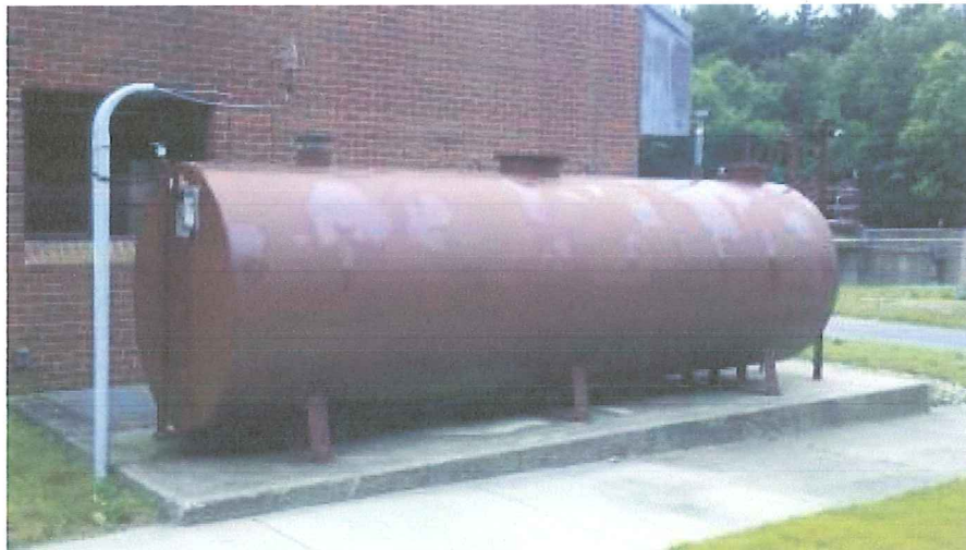
4000 gallon Above Ground Storage Tank Containing #2 Heating Oil
