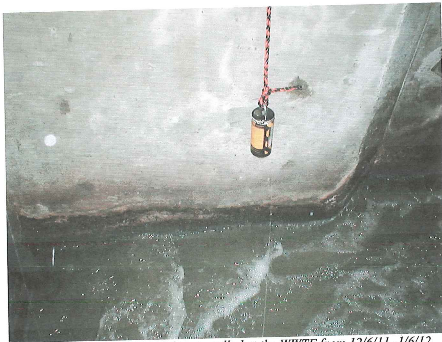
One of the two Siemens odalogs installed at the WWTF from 12/6/11 -1/6/12.
